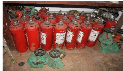
Fire extinguishers lying without installation
